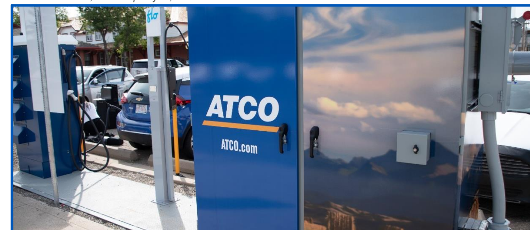
EV Charging Station, Lethbridge, AB
