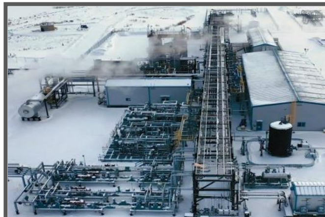
HYDROCARBON STORAGE CANADA 400,000 m 3
