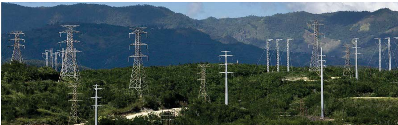
Transmission towers near the Central Costa Sur power plant, Guayanilla, Puerto Rico
