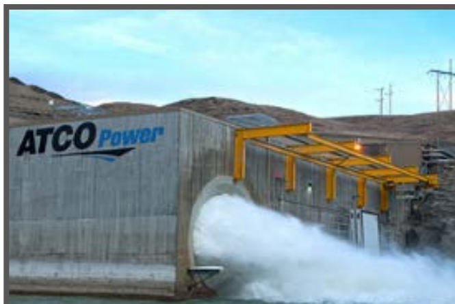
ELECTRICITY GENERATION CANADA 24 MW
