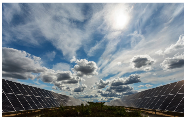
Old Crow Solar Project - Old Crow, Yukon
