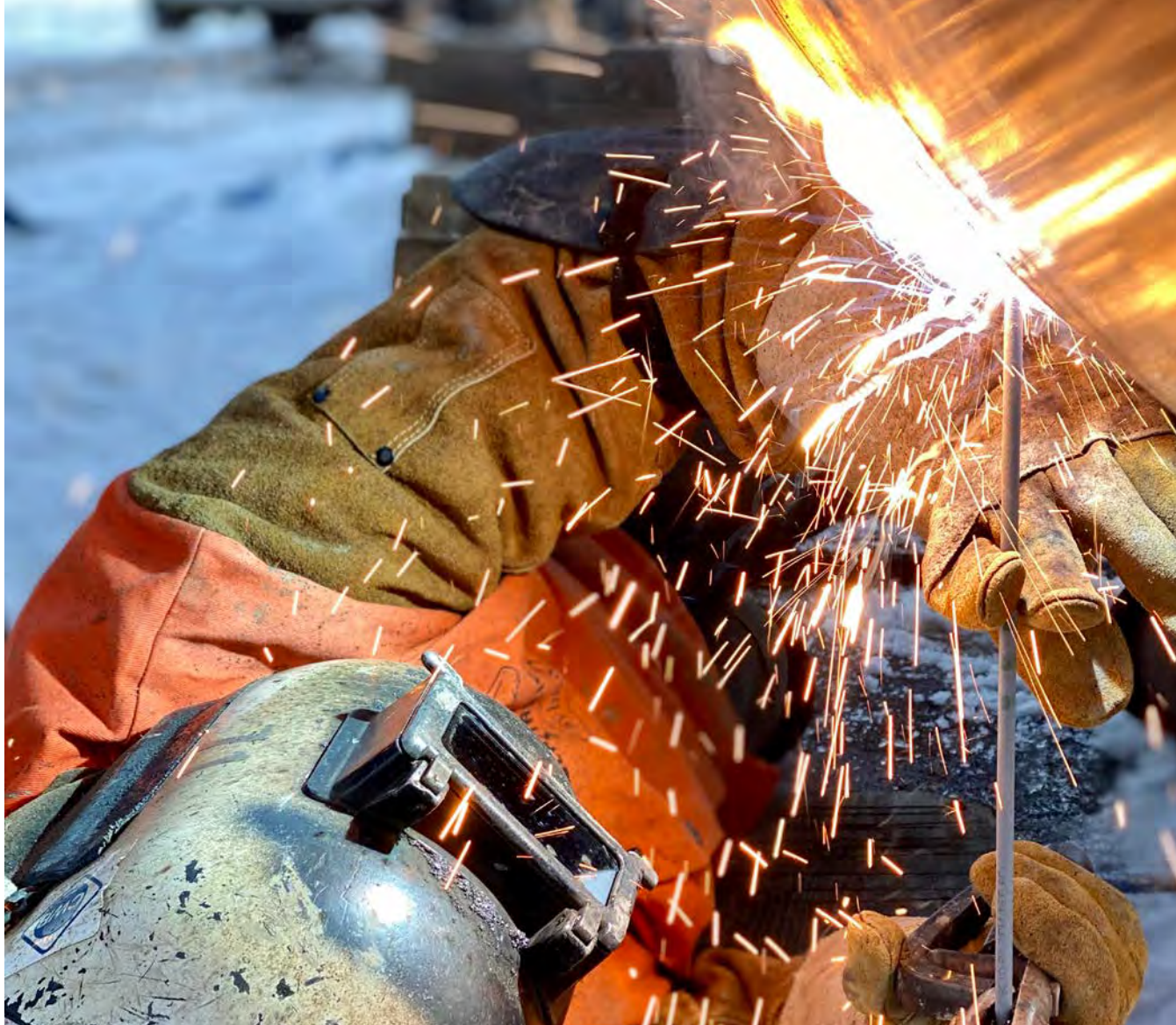
The Pembina-Kepphills Transmission Line directly supports the phasing out of coal-generated electricity, ultimately reducing greenhouse gas emissions with cleaner burning natural gas.
