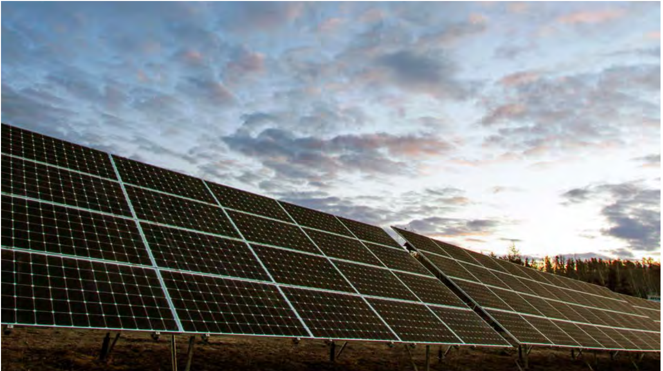
The Fort Chipewyan Off-Grid Solar Project is the largest off-grid solar and storage microgrid project in Canada and will, when fully operational, reduce the Northern Alberta community's reliance on diesel fuel and associated emissions.
