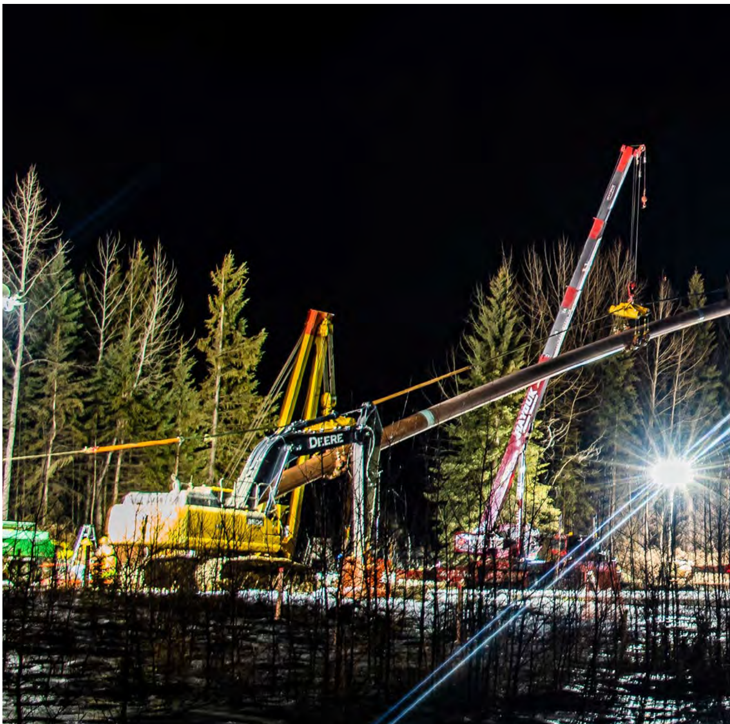
ATCO constructed a new high-pressure natural gas pipeline from its existing Pembina Transmission system near Drayton Valley to its existing Keephills Transmission system in the Genesee area. This pipeline supported the development of natural gas electricity generation in the Genesee area.
