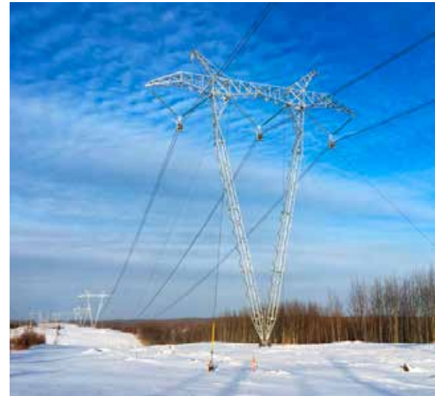
The Fort McMurray West 500-kV Transmission Project, valued at $1.6 billion, was financed in part through the largest public-private-partnership bond in Canadian history.
