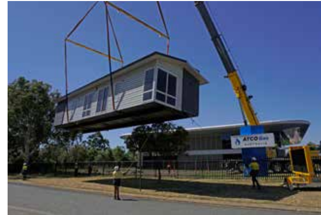
Our modular home being installed at the Clean Energy Hub in Australia is outfitted with the latest in cutting-edge energy technologies and showcases the integrated, customer-centric solutions we can deliver for customers around the world.
