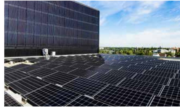
Our people worked collaboratively with Clark Builders to deliver a commercial-scale rooftop solar project at the University of Alberta's Augustana Campus in Camrose, Alberta.
